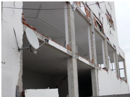
Figure 5: Fallen infill panels reveal beams no deeper than slabs
