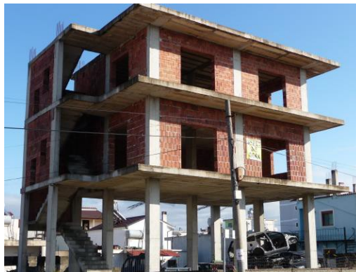
Figure 10: The lower stair landing on the left-hand side is damaged by unseparated stair flights acting as inclined struts in one direction and as elements in bending and shear in the other
