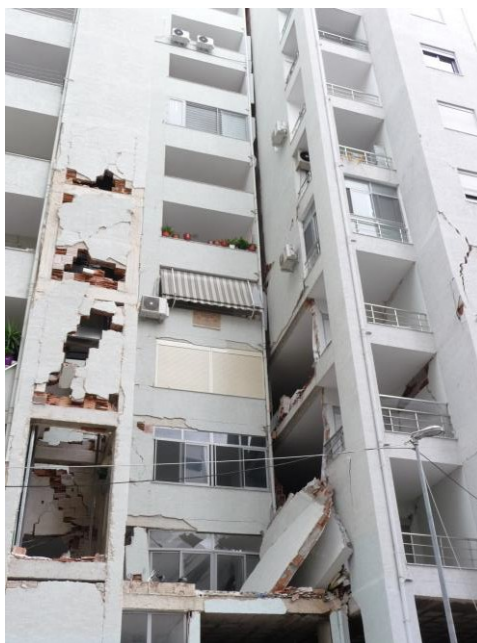
Figure 8: Multi-storey building with extensive wall damage to lower storeys
