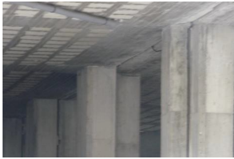
Figure 6: Slab-beams in the first floor of a 12-storey frame building. Note polystyrene rather than hollow clay brick infills.
