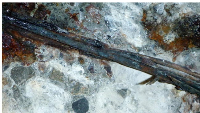
Figure 2 - Visible deterioration of deck unit soffit
