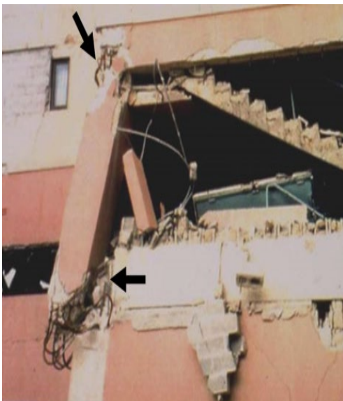
Figure 1: An example of what appears to be an unreinforced exterior joint failure.
