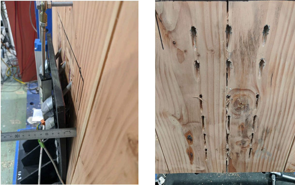
Figure 4: Left: Hold-down bent away from the timber surface by inclined screws. Right: Damaged zone where hold-down was installed.
