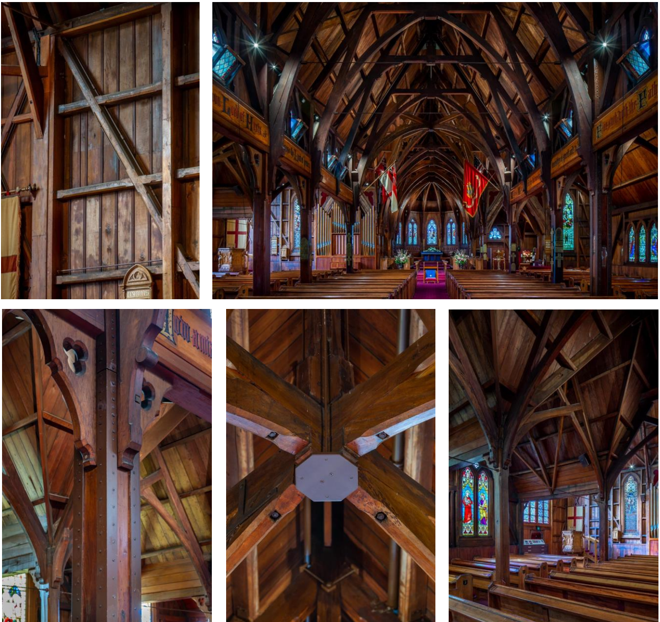
Figure 4: Clockwise from top left: new steel bars in transept wall; new transverse tie rods in aisle; new longitudinal tie rods in north aisle extension; new bearing plate in centre of crossing; repaired column in aisle.
