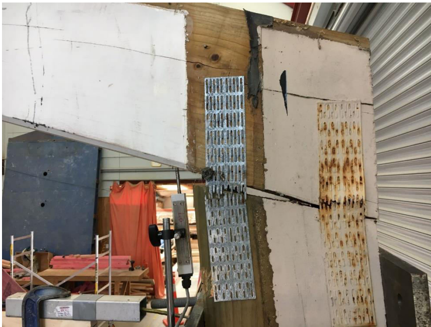
Figure 8 – Failure of the knee joint of the Block R frame (noting the inadequate anchorage length of the gangnail plates)
