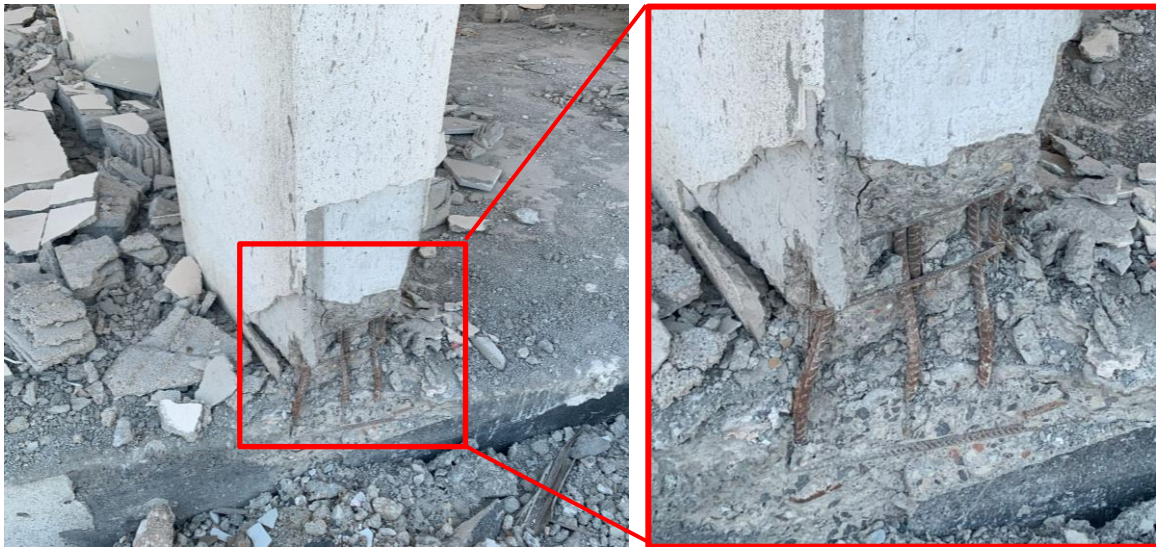
Figure 4: Intentionally bent longitudinal starter bars appearing as 'buckling'.
