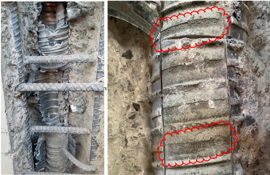
Figure 2: Duct #2 exposed showing partial grout filling (left), Duct #9 exposed showing apparent low-density grout / micro-bubbles in red clouded areas (right)
