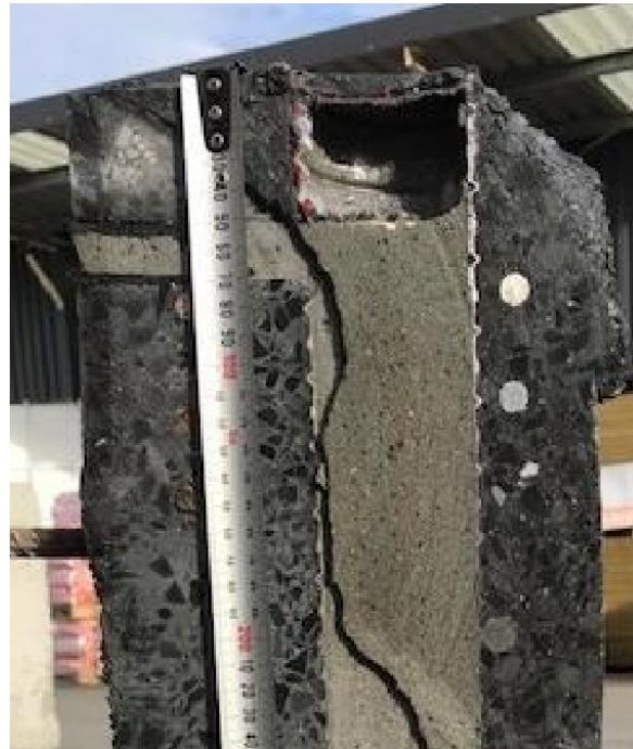
Figure 4: Hollow pocket below top of Drossbach duct (note: jagged line in grout caused by panel dissection process)
