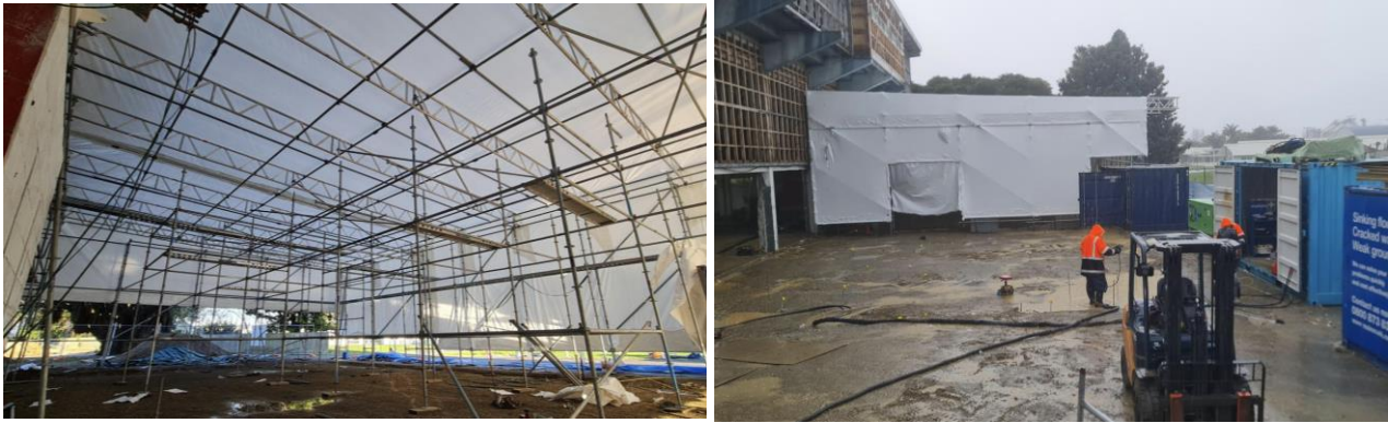
Figure 3 & 4: Images of the Site Setup (Following the construction of the scaffolding - Left, During Stage 1 of Full-Scale works – Right)
