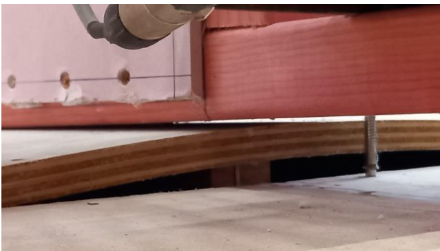
(a) Floor damage
